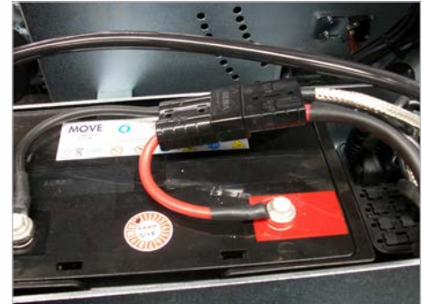
Fig. 39: Main cable battery
